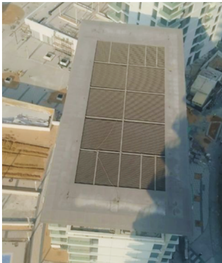
FIBREX CONTRACTING LLC The Cove II" Proposed Mixed Use Development Roof Canopy Steel Structure with ACP Cladding
